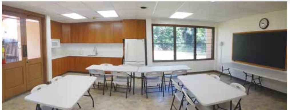
New cabinets, sink, counter, lights and floor tile were all part of the renovations completed in May of the Deacon Joseph W. Borges Sr. Meeting Room.
