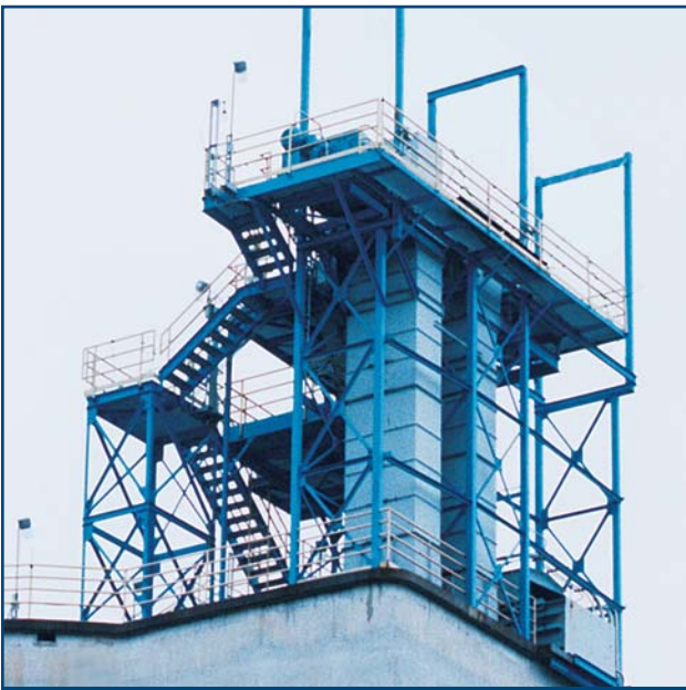
Equipment Support Structures
