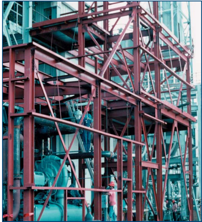
Process Equipment Support Structures
