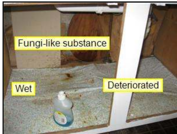
3.4 Picture 1 under kitchen sink
