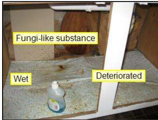
3.4 Picture 1 under kitchen sink
