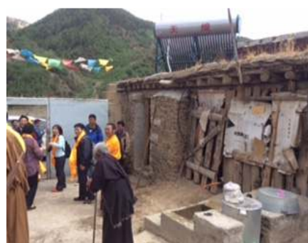
Solar-water heater in Rige Village
