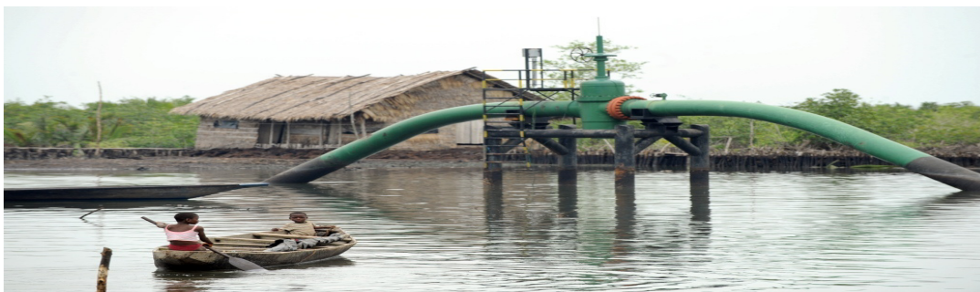
Figure 1: Pipes Fitted with Valves and Gauges in a Pipeline (Source: Shell Nig. Ltd)
